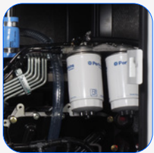
Fuel particle separator filter
