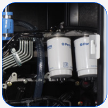
Fuel particle separator filter
