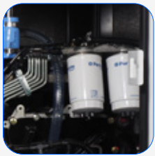
Fuel particle separator filter
