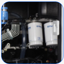
Fuel particle separator filter
