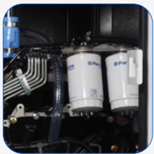
Fuel particle separator filter
