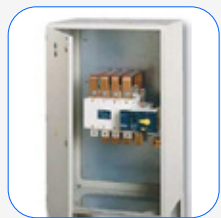
Socomec motorised switchboard
