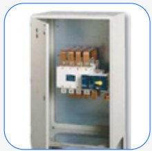
Socomec motorised switchboard
