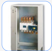
Socomec motorised switchboard
