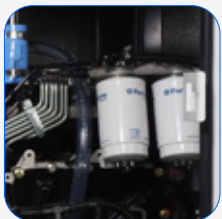
Fuel particle separator filter
