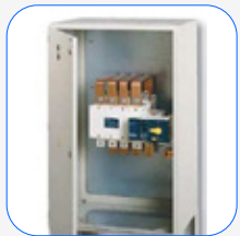
Socomec motorised switchboard
